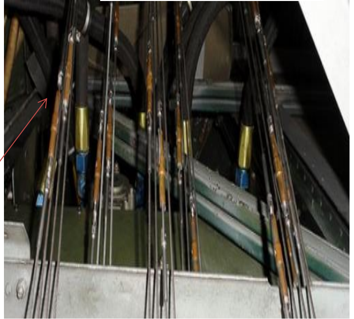
Figure 49-2, control cables, web
